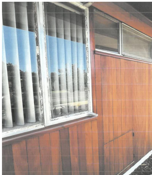
Figure 3 – Redwood siding and window frame and windows in need of repair
