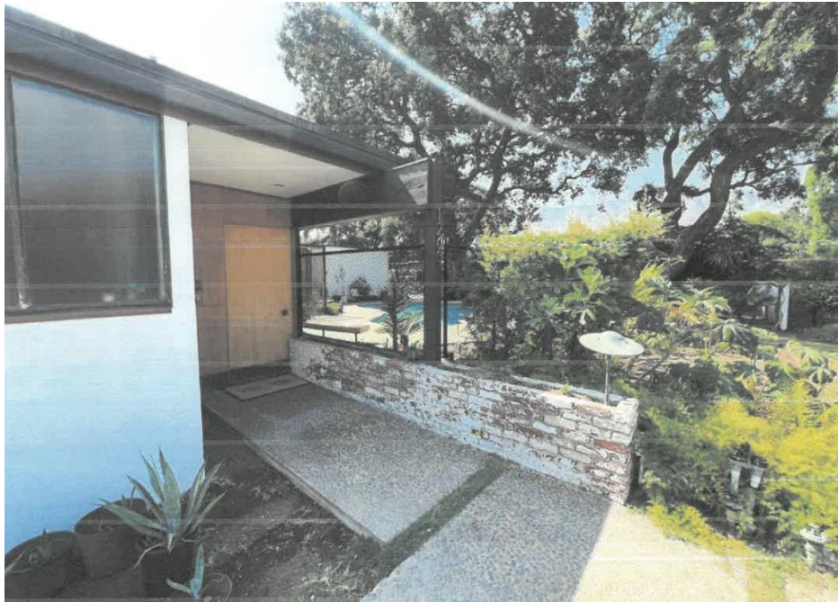
Figure 4 – Planter in need of rehab
