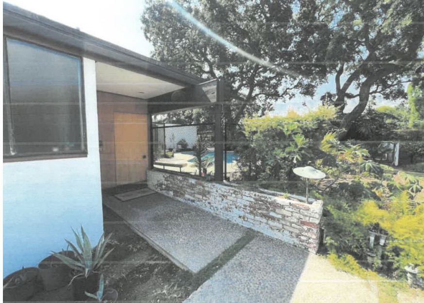
Figure 3 - Planter in need of re-habitation
