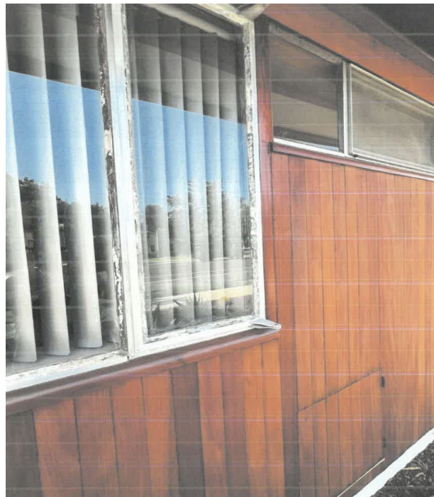
Figure 2 – Redwood siding, window frame and windows in need of repair
